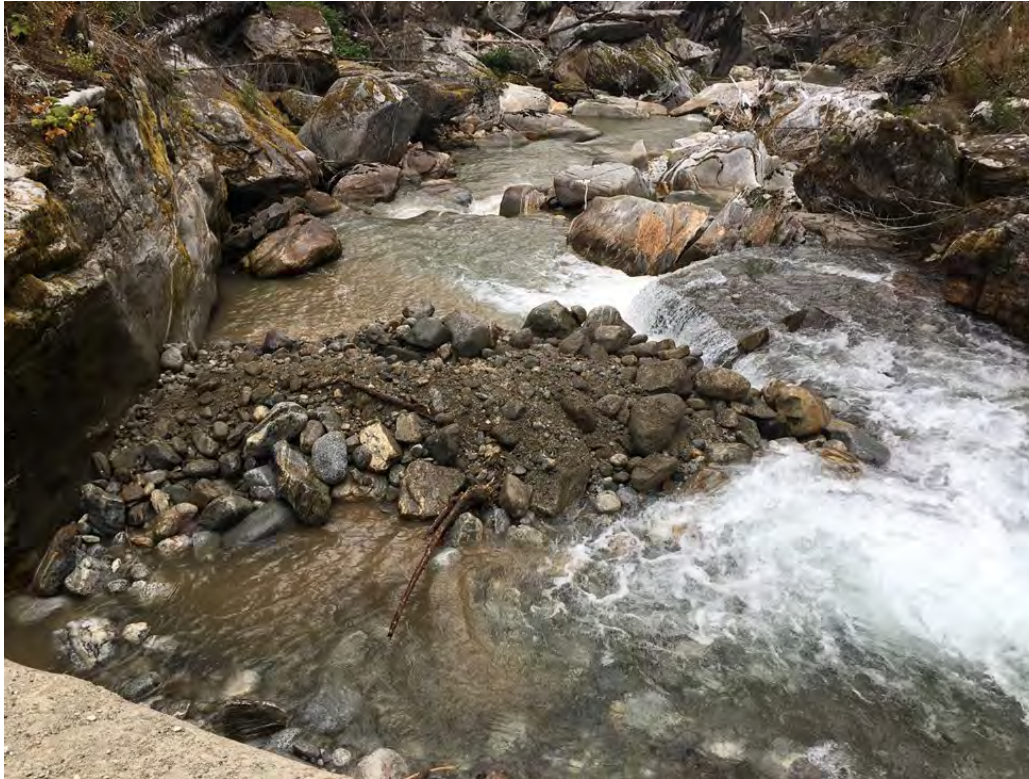
Figure 4.2-3. Material removed from intake pool placed on concrete apron downstream from diversion structure.
