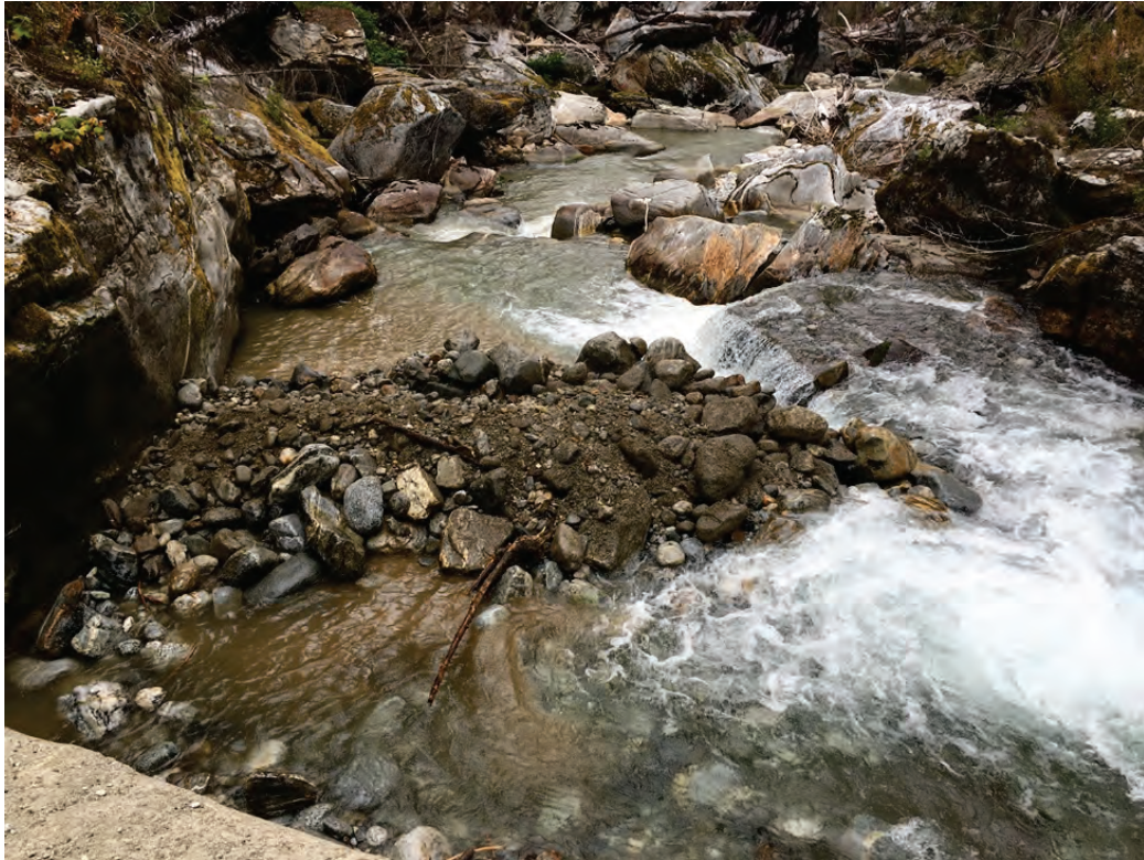
Figure 4.2-3. Material removed from intake pool placed on concrete apron downstream from diversion structure.
