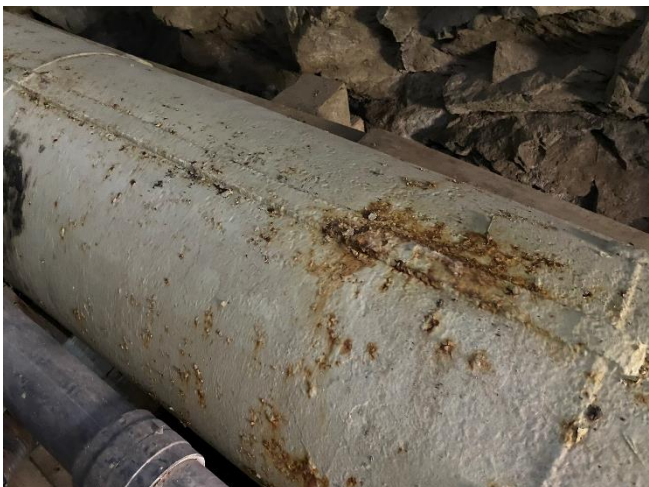
Photograph 11. Minor damaged paint on penstock within adit.
