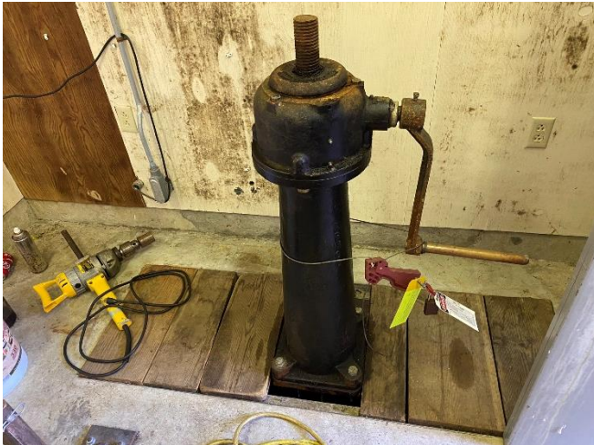
Photograph 3. Control valve located within the gatehouse.
