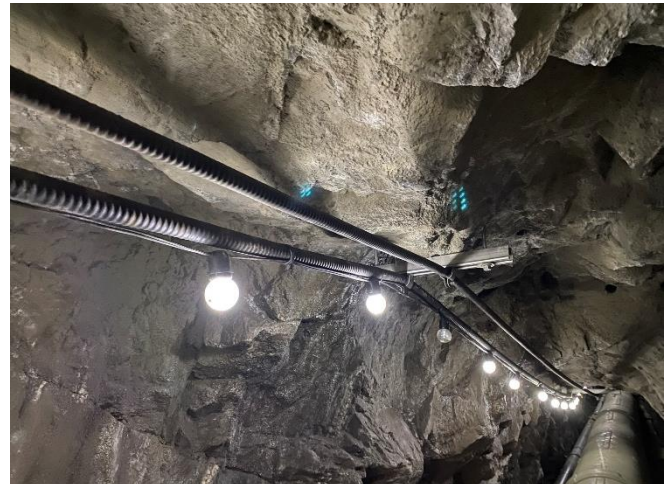
Photograph 10. Conduit along the ceiling of adit.
