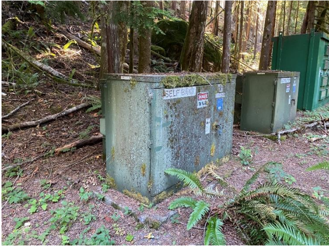
Photograph 199. Transformers located west of powerhouse.
