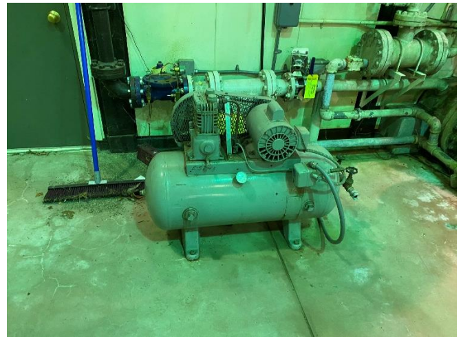
Photograph 16. Air compressor in powerhouse.
