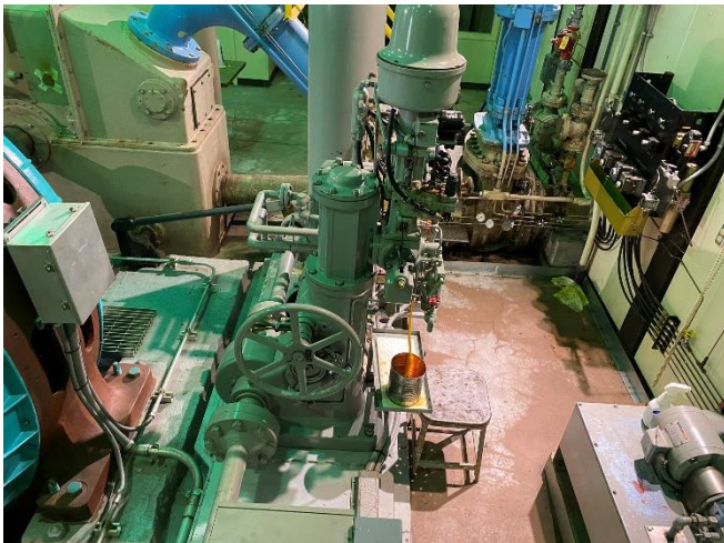
Photograph 15. Hydraulic regulator located on southern portion of powerhouse.
