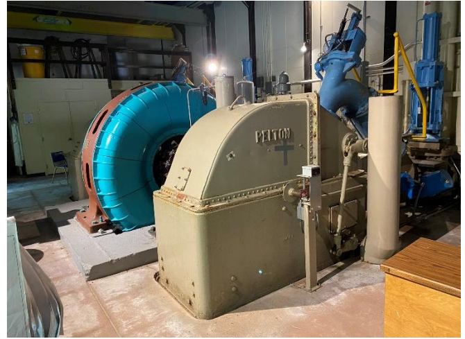
Photograph 14. Turbine and generator in powerhouse.
