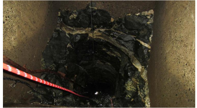
Photograph 8. Vertical shaft entry to power tunnel (from Newhalem Power Tunnel Survey Assessment [Golder 2013]).
