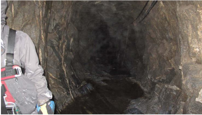
Photograph 7. Representative view of power tunnel interior (from Newhalem Power Tunnel Survey Assessment [Golder 2013]).
