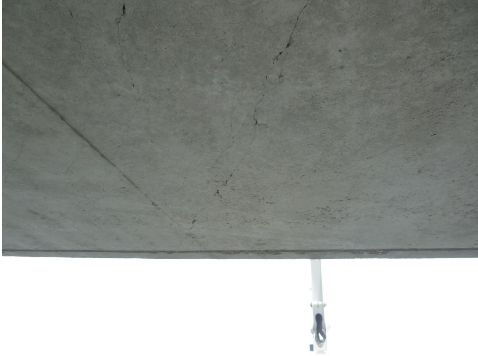
Photo #9 N/E Section, Segment 11, Cracks transitioning to diagonal near web.
