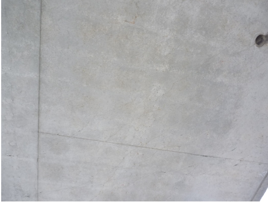
Photo #13 N/W Section, Segment 11, typical cracks
