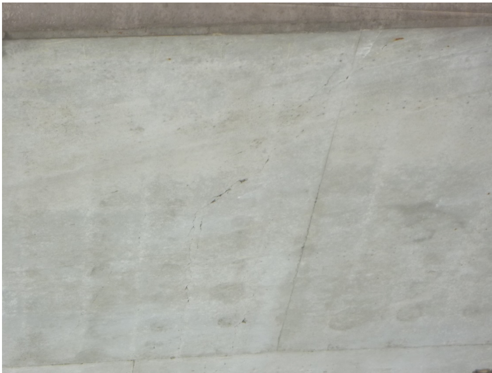
Photo #10 S/E Section, Segment 11, typical crack
