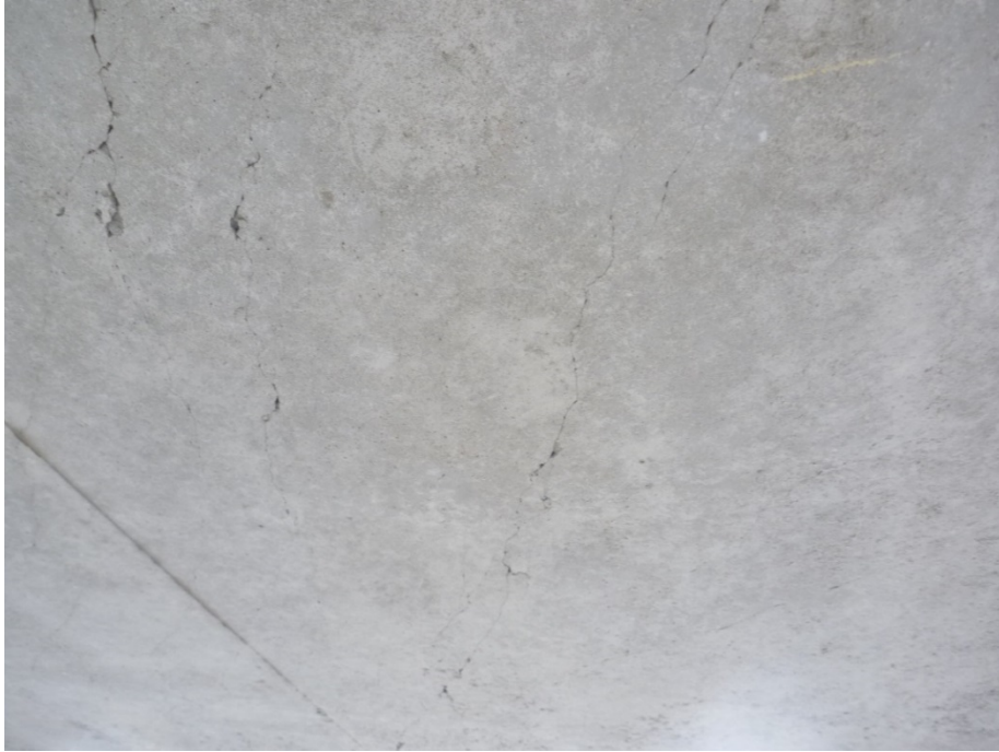
Photo #7 NE Section, Segment 11, typical cracks
