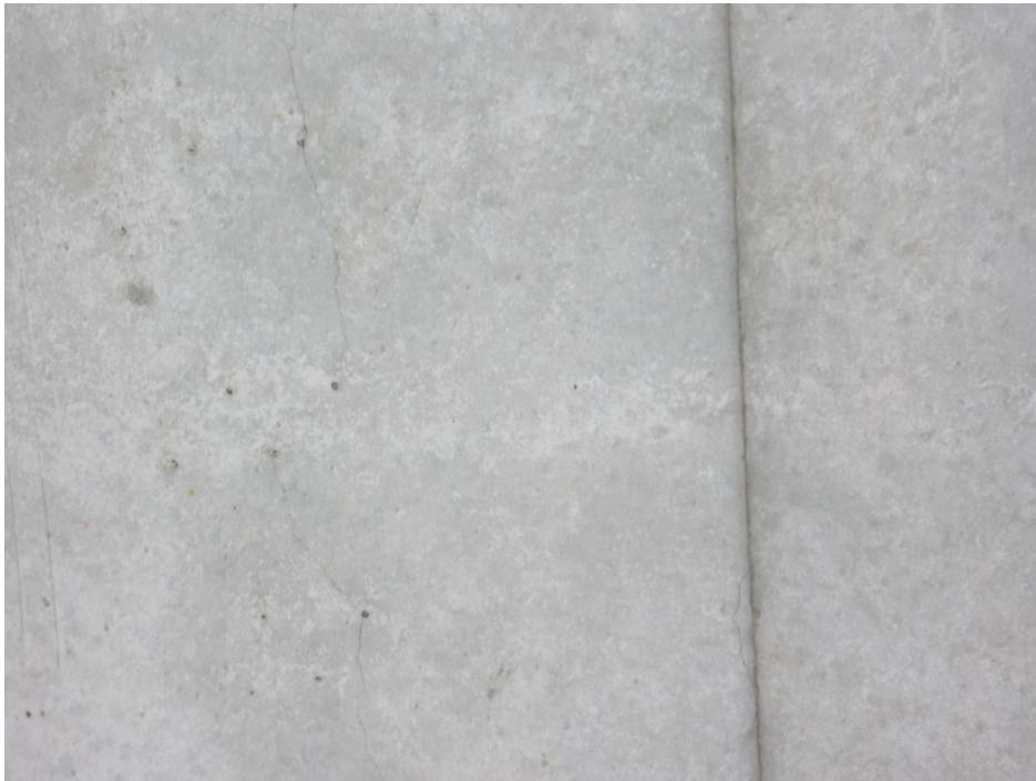
Photo #12, N/W Section, Segment 11, typical cracks
