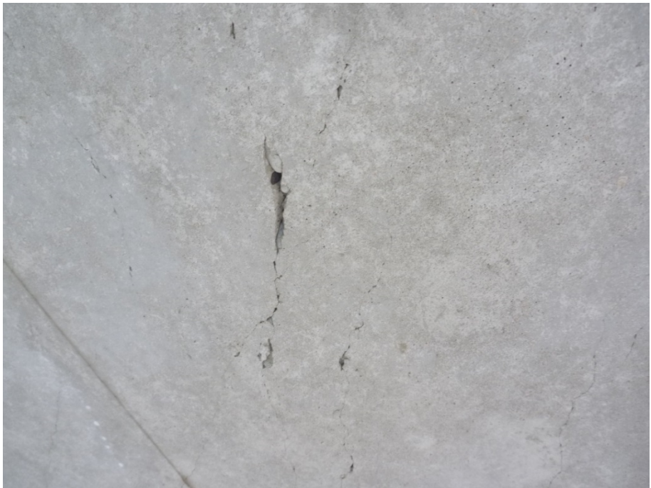
Photo #8 NE Section, Segment 11, typical cracks
