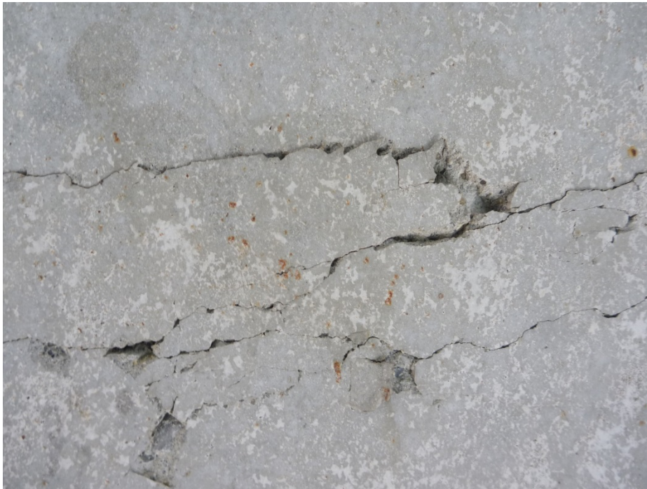
Photo #5 N/E Section, Segment 11, close up of transverse crack
