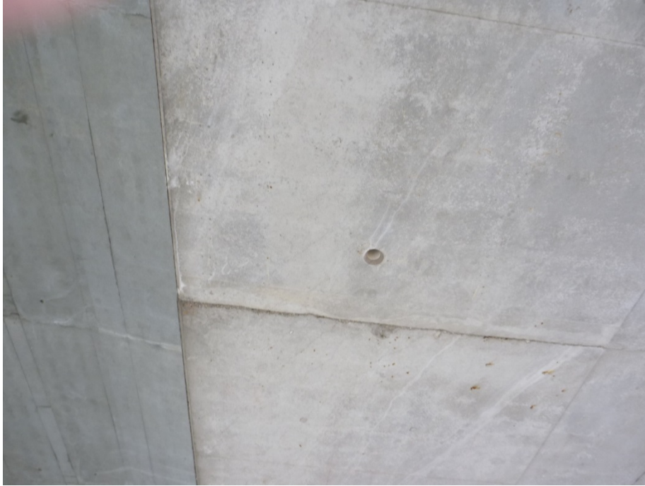
Photo #3 N/E Section, Segment 11 – diagonal cracks spanning into segment 12
