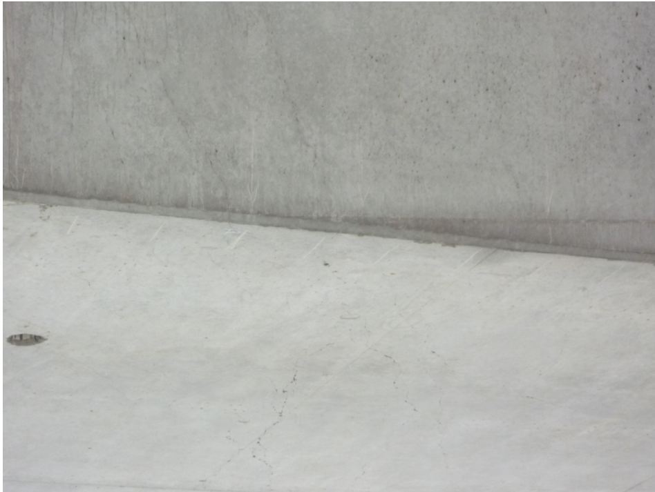
Photo #12 S/W Section, Segment 11, close up of continuous cracks into web
