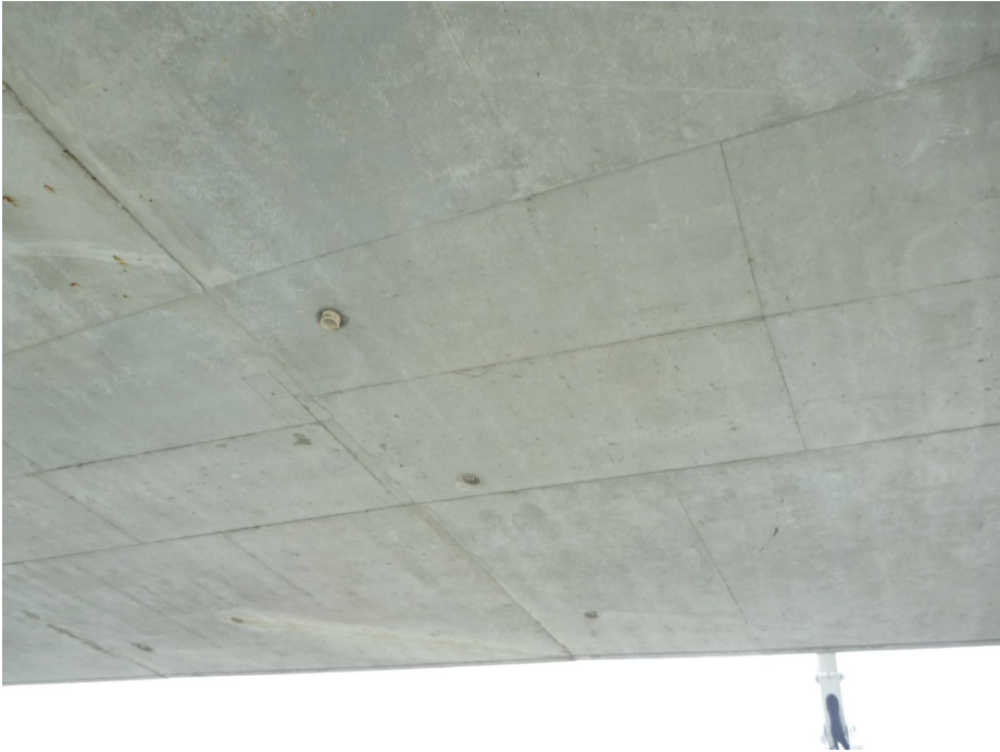
Photo #2 N/E Section, Segment 11 – transverse crack transitioning to diagonal
