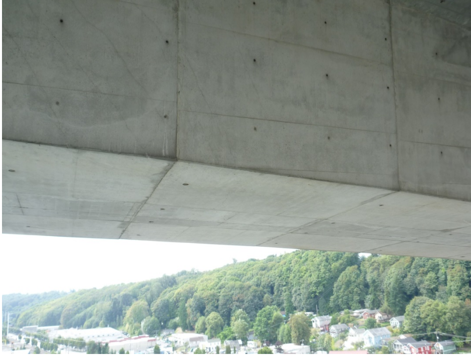
Photo #11 S/W Section, Segment 11/12, continuous cracks into web
