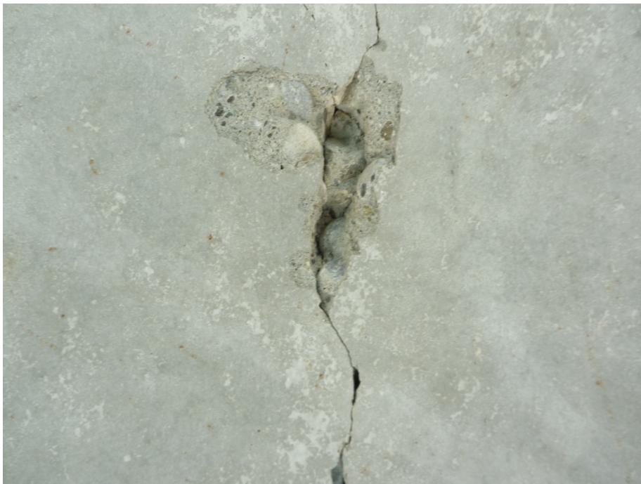
Photo #4 N/E Section, Segment 11 - close up on transverse crack with spalling, 5"x1"x3/4"
