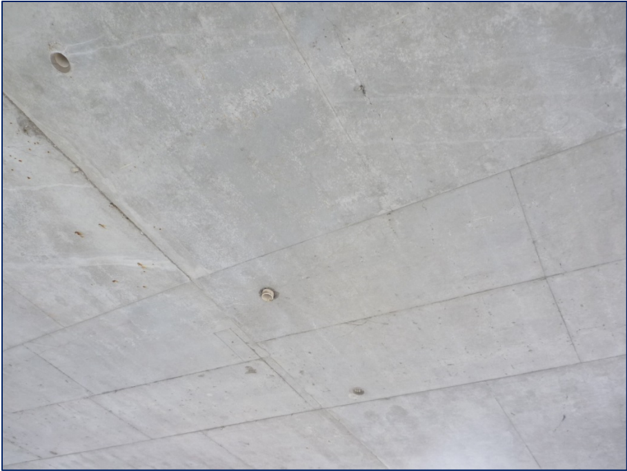
Photo #1 N/E Section - Prominent transverse crack
