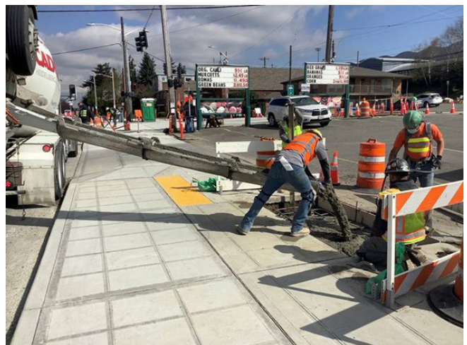
15th Ave S and S Columbian Way crossing improvement for Mercer Middle School
